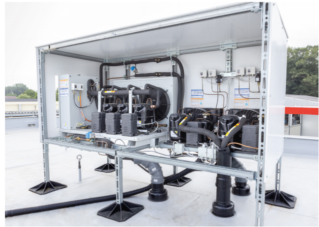
R-1234yf centralized system and two stand-alone LT units with R-454C.
