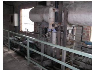
Fig. 2 Receiver and Witt Refrigerant Pump
